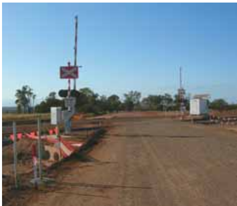
Looking south towards Rolleston - the boomgates and flashing lights have now been installed at the Rolleston - Comet Road intersection with the new Bauhinia Regional Rail line.
