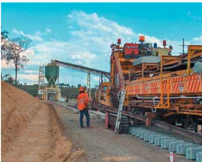
The final sleepers are laid on QR's Bauhinia Regional Rail line at Rolleston Mine's coal loading facility.
