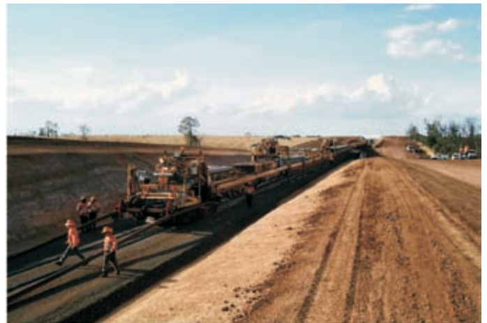
Track laying commences at the northern end of the Bauhinia Regional Rail Project.
